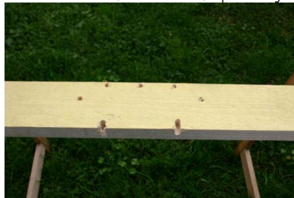
After marking the screws of the beam, drill the locations for mount the wood board.
