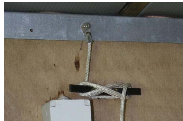
View on the nylon rope attached to an electrical terminal
